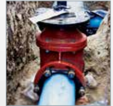
Water & Sewer Lines
