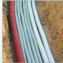
Electric Power Lines
