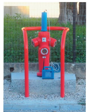
Fire hydrant injection
